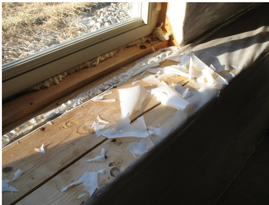
Figure 1: Degradation of polyethylene barrier membrane due to UV exposure
