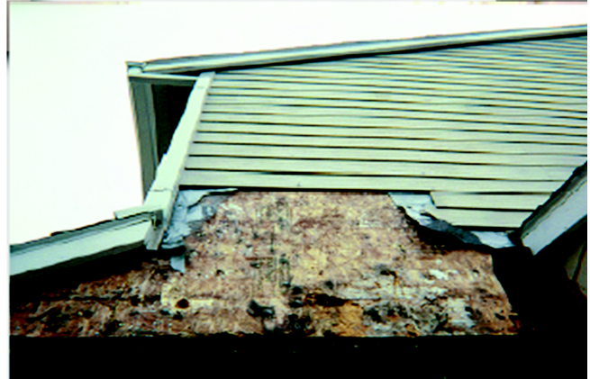
Figure 1 Failure building envelope system with a "breathable" type WRB.
